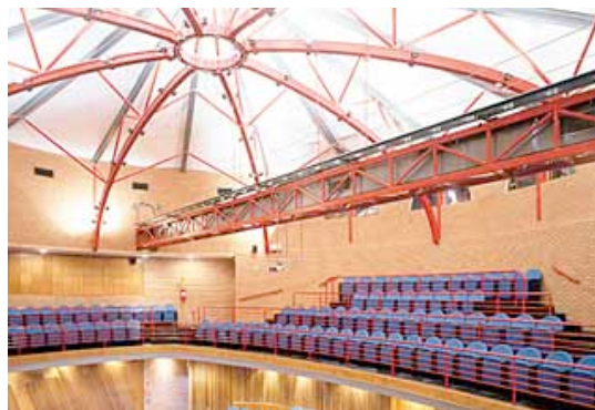
Coverage metal space under massive stone and acoustic insulation lateral prevent the entry and exit of sounds
